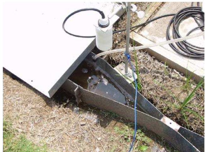
Ultrasonic modules (ISCO 710) mounted over each Parshall flume used ultrasonic reflection to measure water levels.
