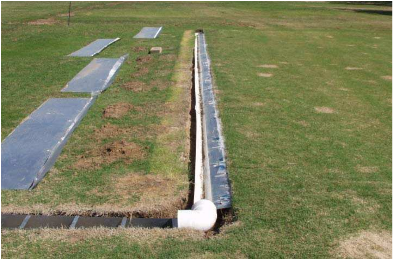
Covered troughs collected runoff water from each plot and channeled it through calibrated Parshall flumes by gravity flow.
